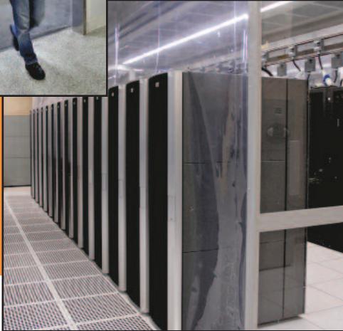
Data centers and computer rooms.
